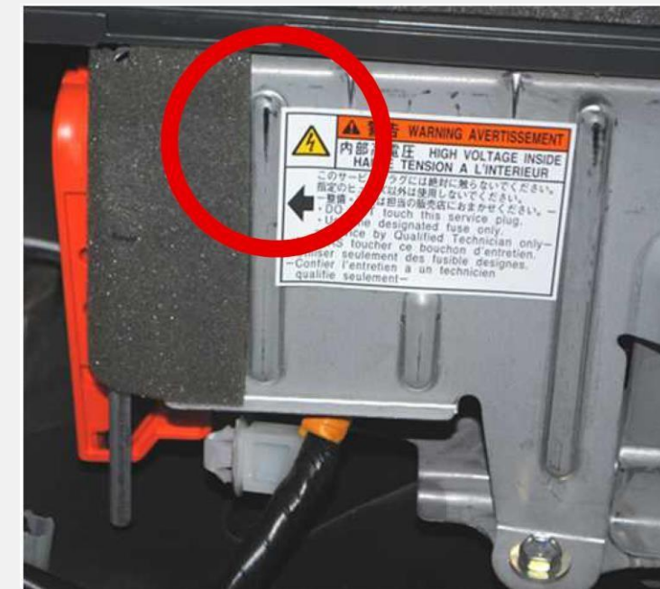
Warning label on Battery
